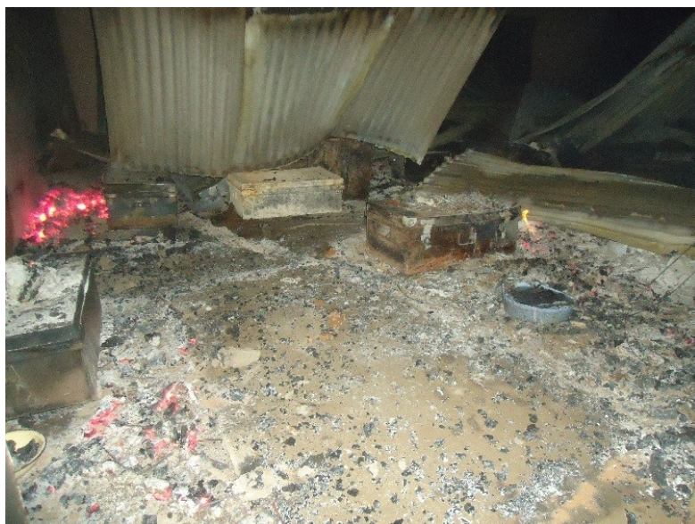
Photo: Joseph Amunya A section of the burnt dormitory
