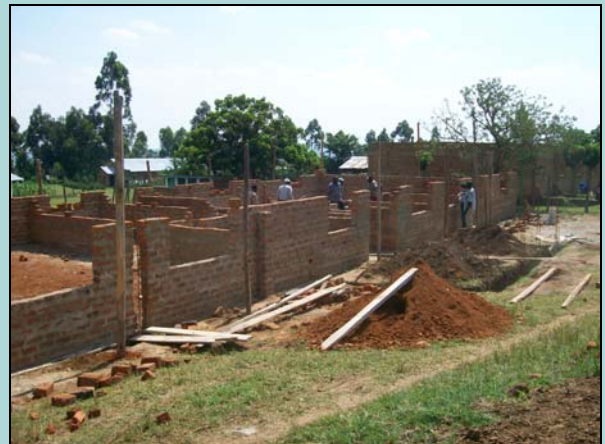
Unfinished administrative block, due to lack of funds
